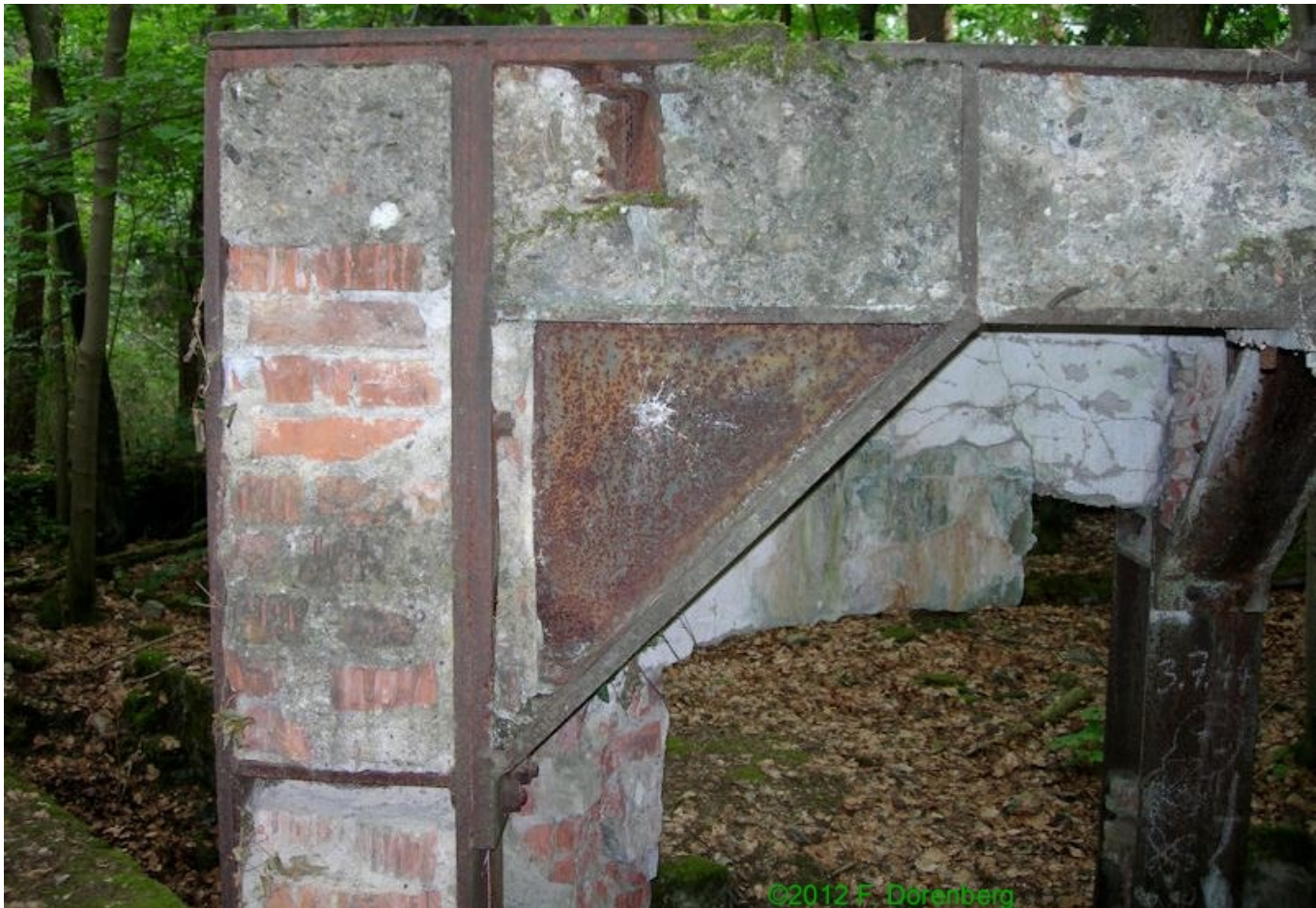
Fig. 42: Details of the steel support structure of the "Bernhard" Be-14 ground station
