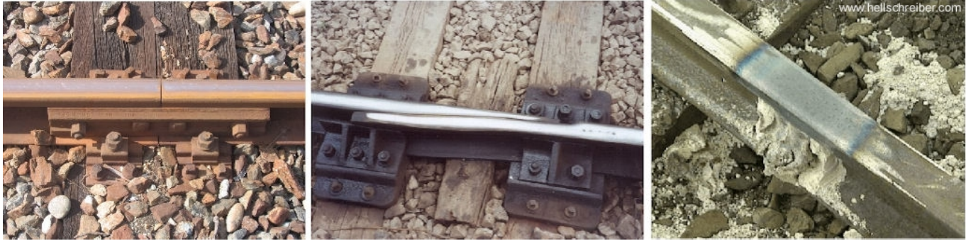
Fig. 19: Three standard types of rail joints (left-to-right: conventional joint, expansion joint, seamless joint)
