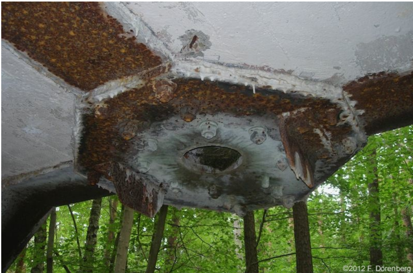
Fig. 43: The octagonal mounting plate against the ceiling - with mounting brackets to suspend equipment
