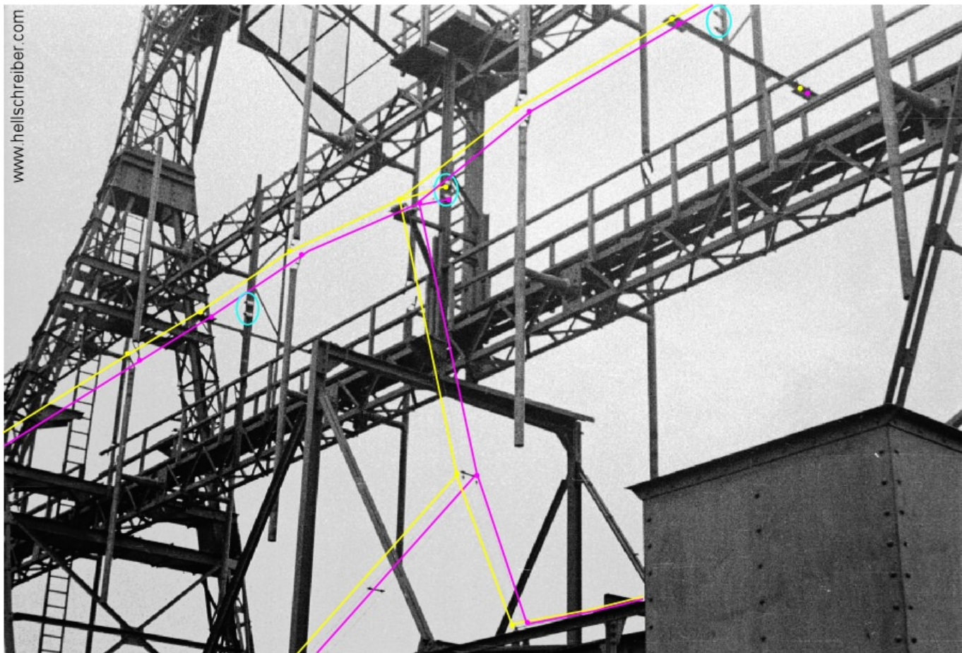
Fig. 124: Antenna feedline routing from transmitter at Bredsted
