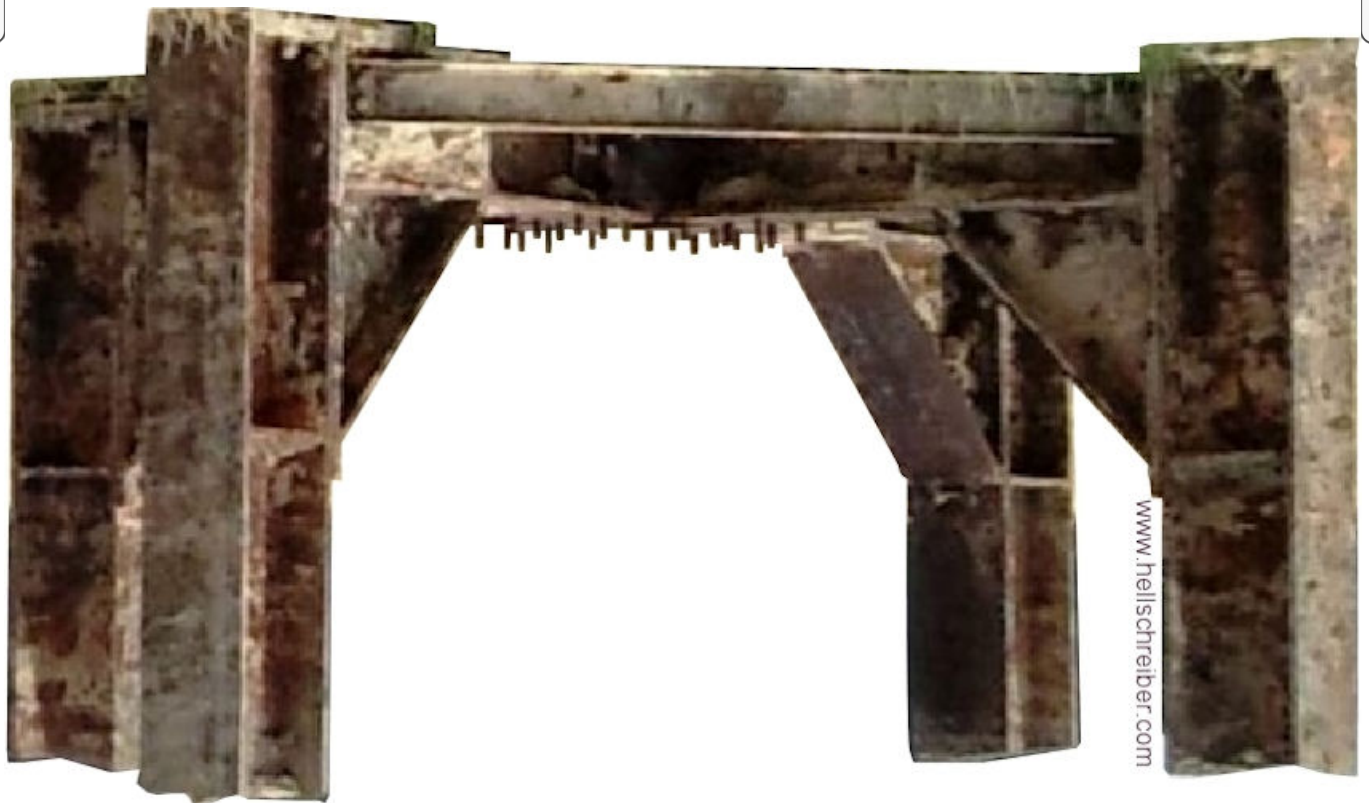
Fig. 45B: The remains of the steel structure at Be-12 , after destruction of the building in 2015
