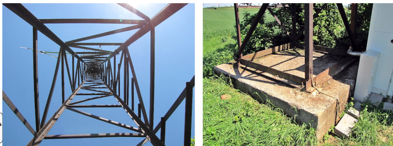
Fig 181: Looking up inside the monitoring antenna mast, and the base of the mast at Be-11 Trzebnica/Trebnitz
