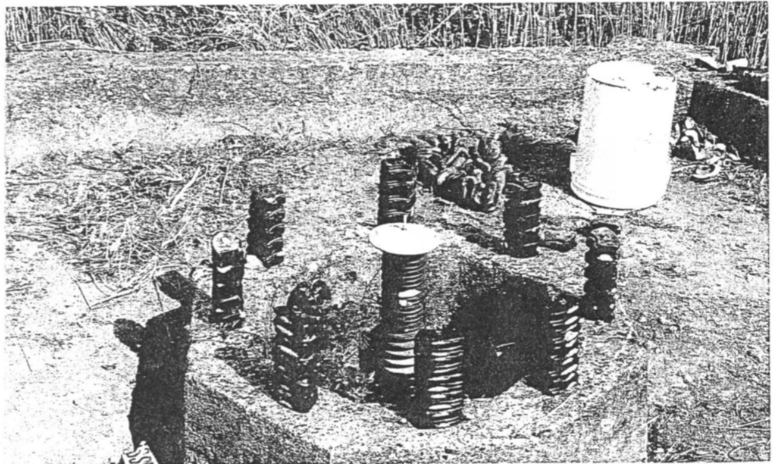
PTB/fig. 37 D : unknown shack Foundation Series coil insulators stacked as in use
